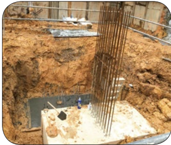
Figure A: Site photo of improper slope.
