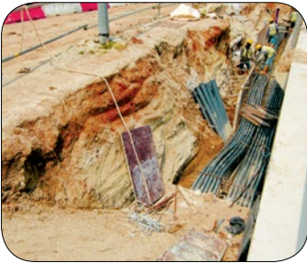
Figure H: Site photo of unsafe access/egress.
